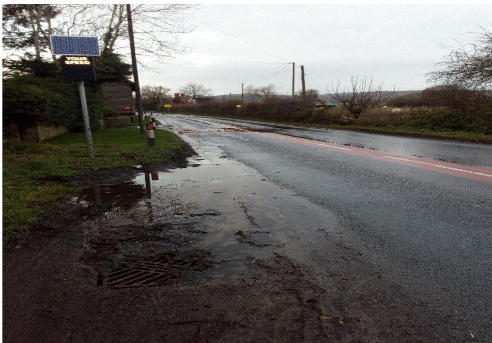
Fig.8 B4362 looking towards the proposed development and the junction with Kings Road illustrating surface water issues already existing.
